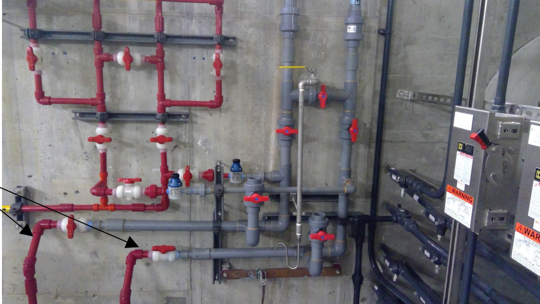
Temporary 1.5-inch CPVC Piping (A-Side UV Room Valve Station)
