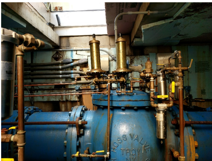
Figure 1: Interior of Nonantum Road PRV Vault
