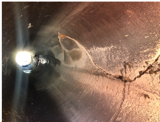
Cracked section of Section 79
