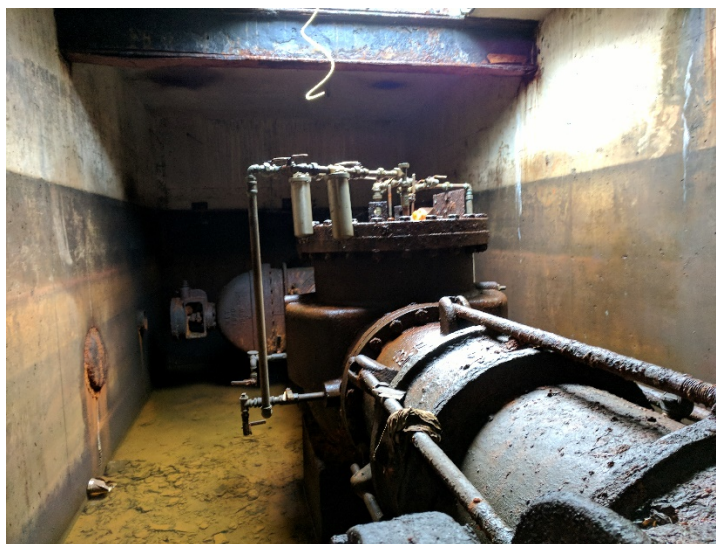
Figure 2: Interior Mystic Valley Parkway PRV Vault
